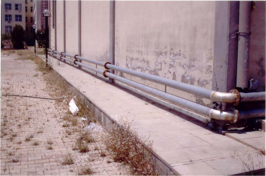
Figure 5.23: The view of second pipeline system.
