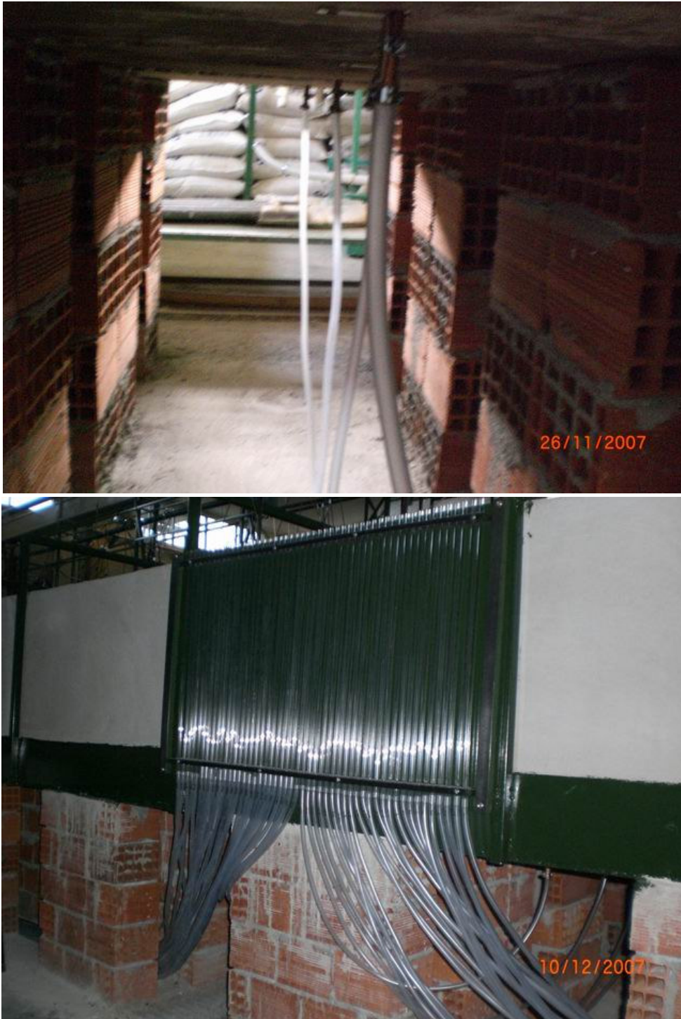
Figure A.14 The panel of piezometers for reading the water levels
