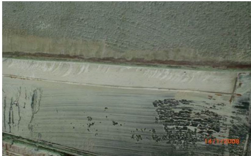
Figure A.25 Cutting of the metal sheets and slotting of the wall in order to apply insulation material
