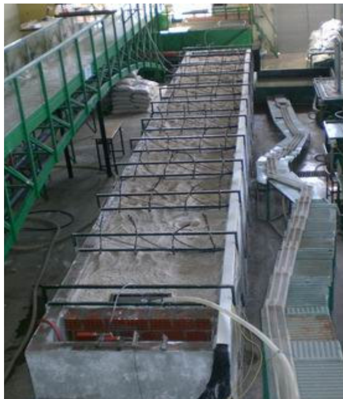
Figure A.23 General view of the channel with armoured cables
