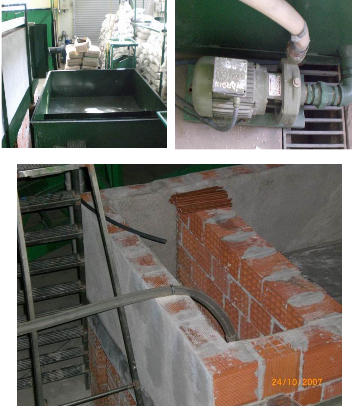
Figure A.11 The water supply tank
