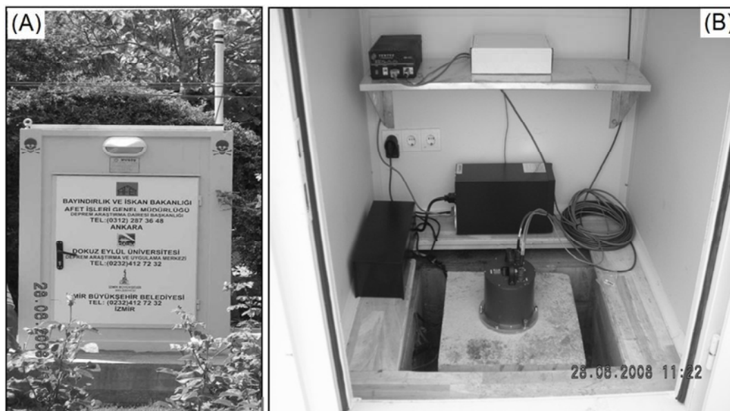
Figure 4.3 Typical installation of IzmirNet strong-motion network. (A) Recording stations are housed in the standardized small galvanized hut as shown at KSK location. (B) Inner view of a container with a typical installation of free-field station. CMG-5TD built-in system is mounted on a prefabricated concrete block.
