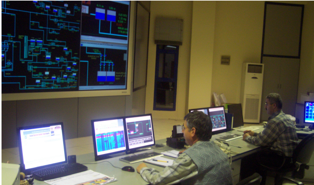
Figure 3.3 The SCADA center of the İZSU Water Distribution System, İZMİR
