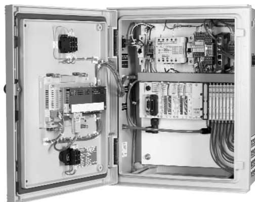
Figure 4.48 A control cabinet
