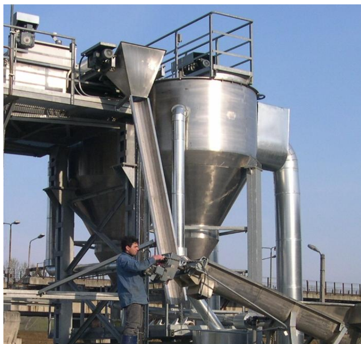
Figure 4.3 Grit classifier run cycle arrangement during commissioning.
