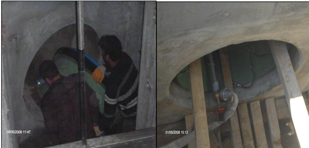
Figure 4.2 Pipe impermeability test. Installing the test valve and supporting it with wood blocks. Test valve was connected to hydrant water and other opening of pipeline is closed by test balloon. Then line was filled with water and waited definite time. Pressure is checked by manometer attached on test valve. Piatra Neamt Wwtp-Romania
