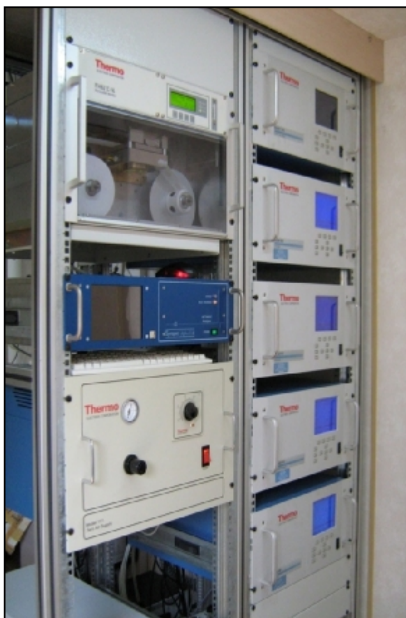
Figure 4.4 The equipments used in the station.
