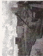
The site is being cleared making way for the new King's Place building
