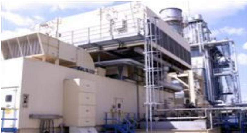
Figure 4.8 Ataer energy power plants in IAIP
