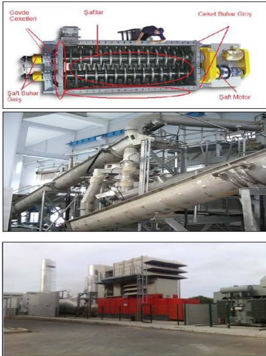
Figure 2.12 Pasakoy WWTP Sludge Drying Unit and Cogeneration Plant
