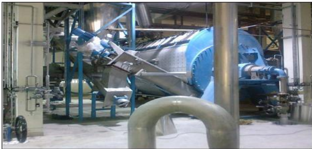
Figure 2.13 Atakoy WWTP Sludge Drying Unit an a view of a dewatered sludge cake and dried product (the upper pics).
