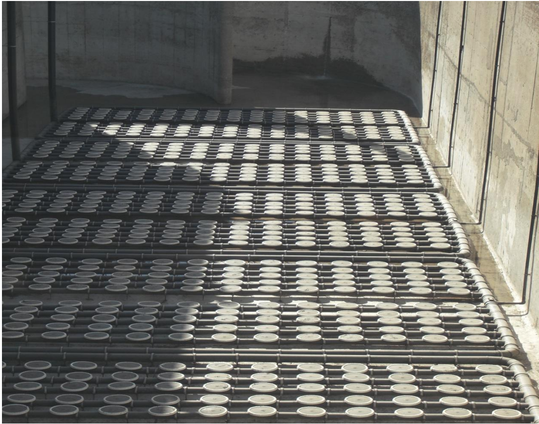
Figure 6.6 View of diffusers placed in the bottom of oxidation ditch.
