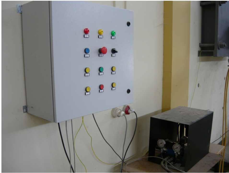
Figure 3.40 Control panel of actuator
