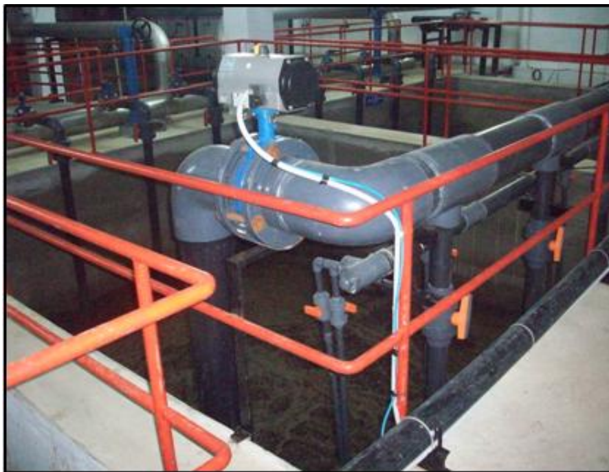
Figure 3.13 MBR automation system
