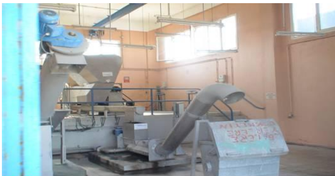
Figure 5.13 Belt-filter press of Dalaman domestic WWTP.
