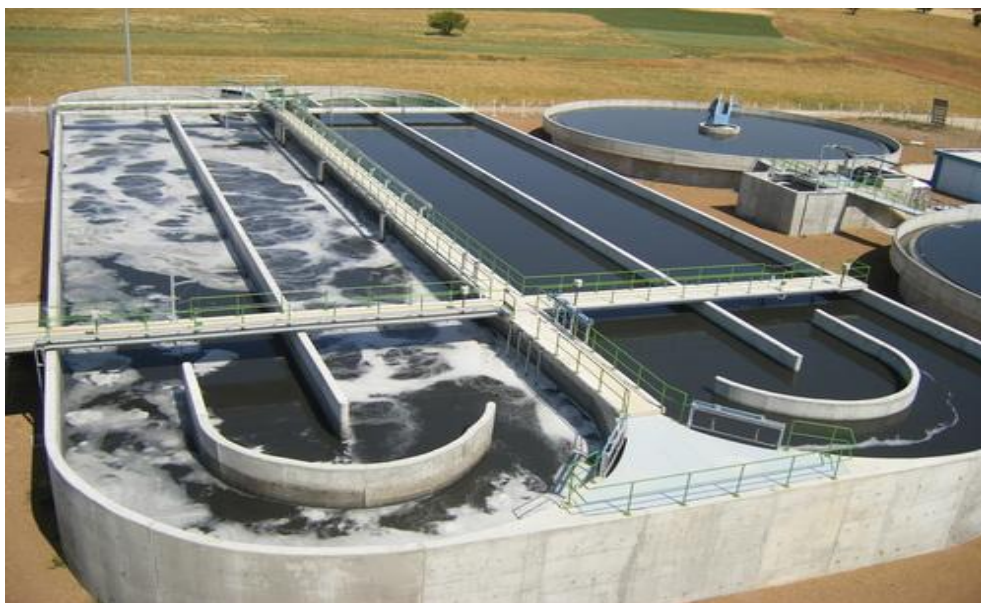
Figure 5.19 Usak wastewater treatment plant.
