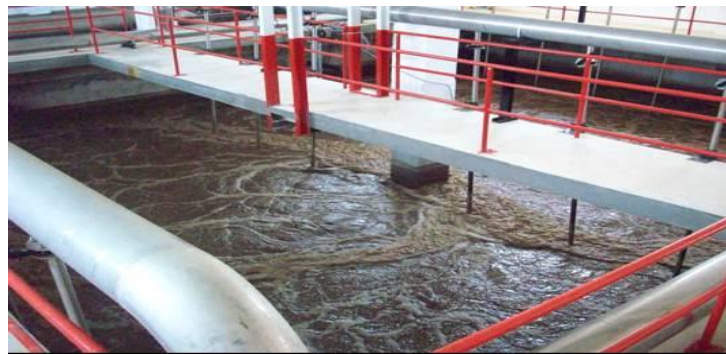
(b) Activated Sludge Tank with Submerged Membrane Unit
