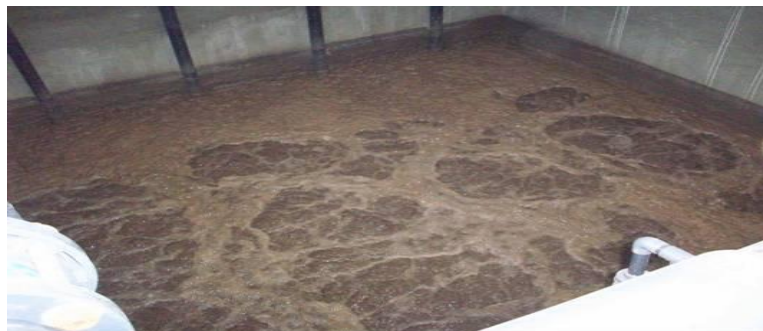
(c) Activated Sludge Tank with Submerged Membrane Unit
