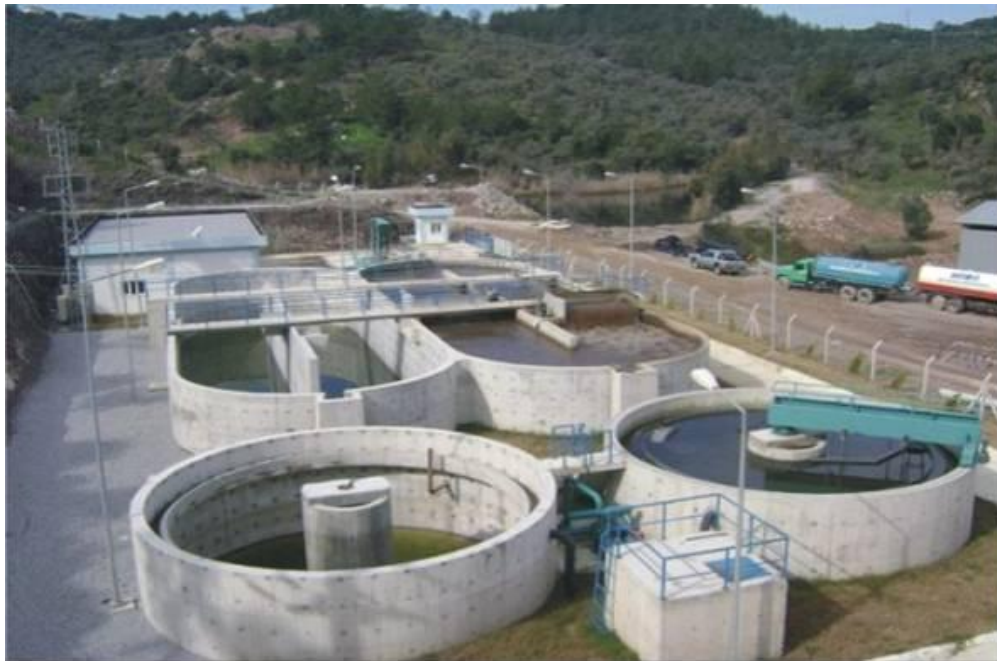
Figure 5.14 Güllük Municipal WWTP.
