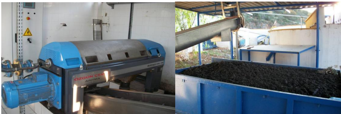
(c) Decanter centrifuge and sludge collecting systems of Bitez WWTP
