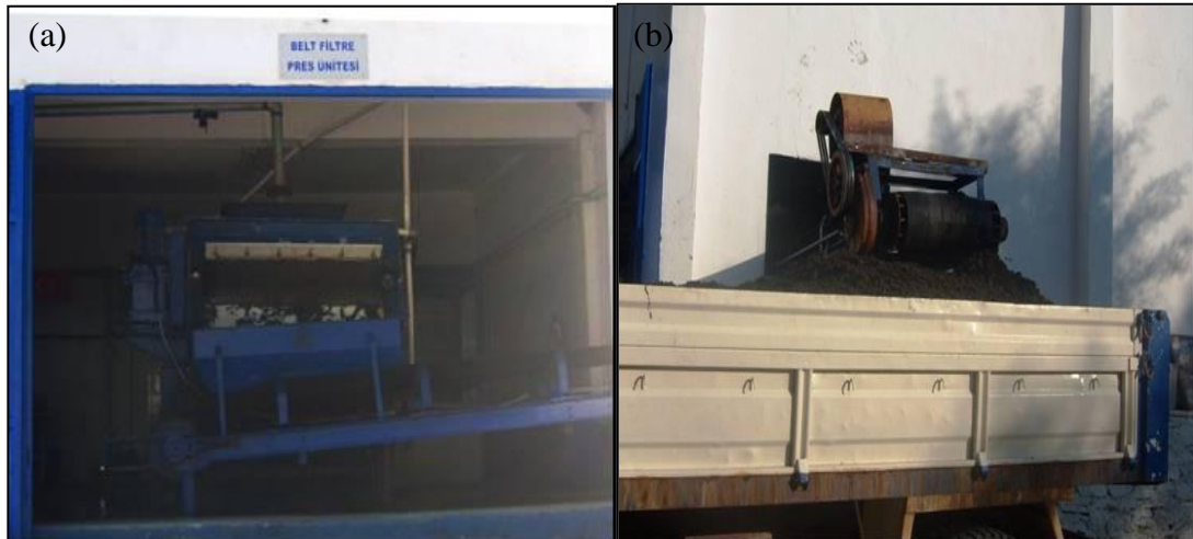
Figure 5.8: (a) Belt filter and (b) Sludge collection units of Bodrum WWTP, İçmeler-Bodrum/Muğla
