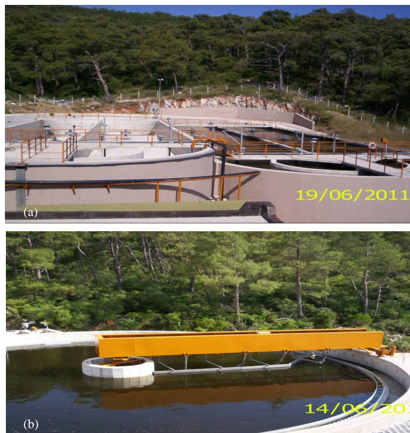
Figure 5.16 (a) Denitrification unit, (b) Sedimentation tank of Golturkbuku wastewater treatment plant.
