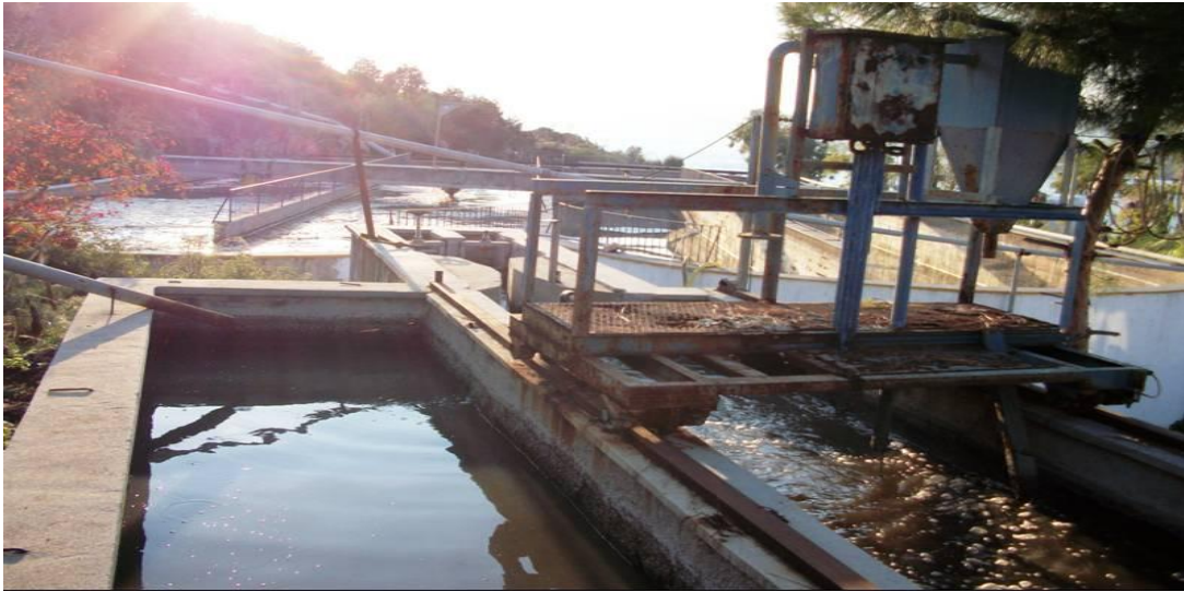
(a) Pretreatment unit of Bitez WWTP (Grit chamber)
