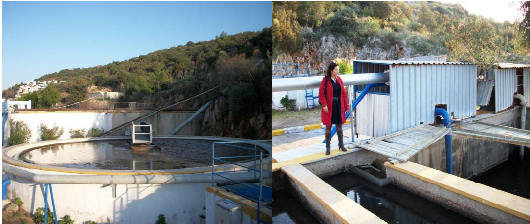
(b) Sedimentation tank and outlet structure units of Bitez WWTP
