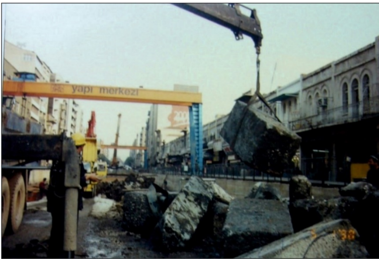
Figure 2: Izmir, Çankaya, Fevzi Paşa Bulvarı. Metro excavation 1997-2000. Lifting of the ancient items discovered during the excavations.
