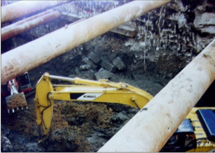
Figure 1: Izmir, Çankaya, Fevzi Paşa Bulvarı. Metro excavation 1997-2000. In the background some ancient blocks are visible.
