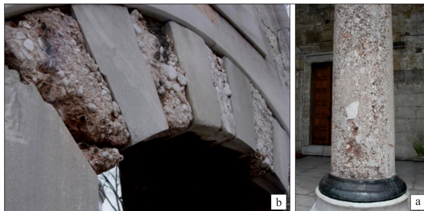
Figure 15: Degradation and destruction of the Hereke puddingstone used in the gate arch of Süleymaniye Mosque (a) and in the portico column of the inner courtyard of the Sultanahmet/Blue Mosque (b) (Photos: Anđı 2010a; 2010b).
