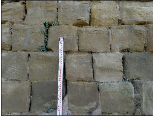
Figure 3: Detail of the Islamic wall of Wasqa. Ashlars (0.3 x 0.3 x 0.9 m) in header bond style wall. (Photo: J.A. Cuchí).
