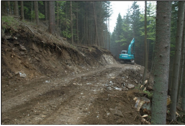
Figure 2: The new forest road built in 2011, cutting into the debris piles of the new Roman marble quarries on the Kalkkogel, view from east (Photo: A. Hassler).
