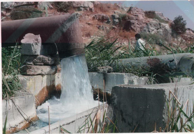
Photograph 5. Corrosion effect of ground water.
