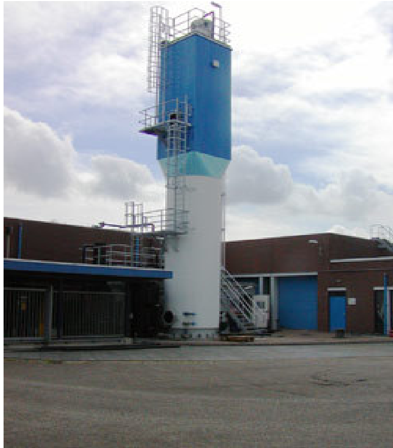
Figure 2.12 The first full scale anammox reactor, Rotterdam, the Netherlands. It works at design load and removes over 500 kg N/day. (the anammox online resource- http://www.anammox.com/application.html )
