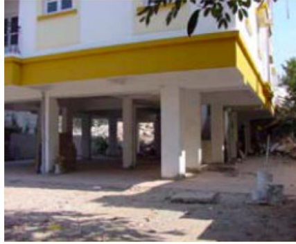
Figure 4.14 Typical building with a soft ground storey in India (EERI 2001).
