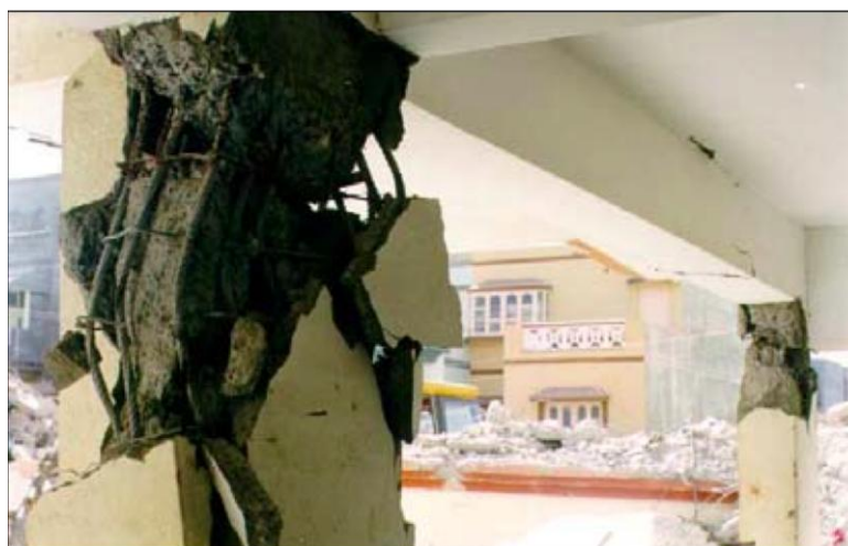
Figure 2.3 Shear failure of a reinforced concrete column (EERI 2001).
