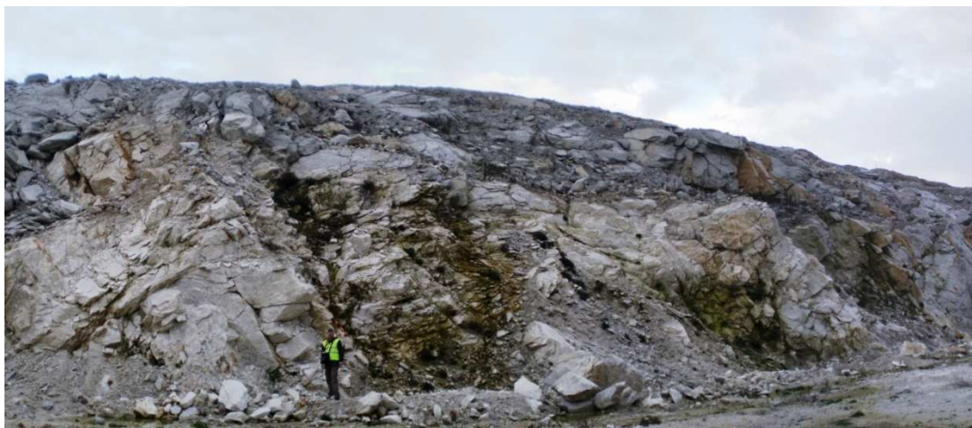
Figure 6.6 Plant growings and damp areas along the shear joint zones.
