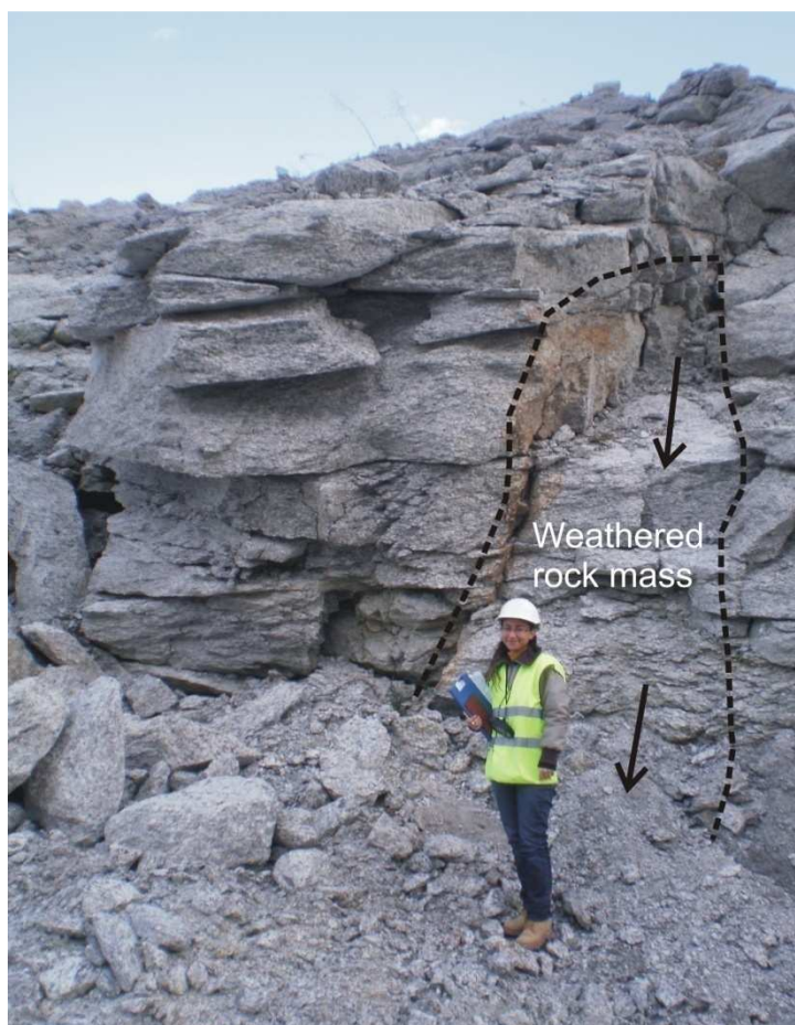
Figure 6.3 A view of seepage point into the crack opened by rock movement and planar foliations in the orthogneiss rock mass.
