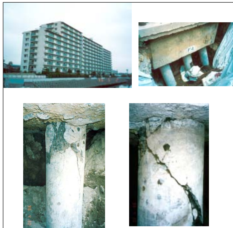
Figure 1.2 Pile damage near ground surface (Kobe Earthquake, 1995)
